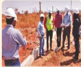
4. Earth Resistance Testing
