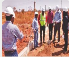
4. Earth Resistance Testing
