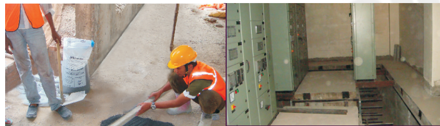
Anti-static flooring in Marconite at RRVPNL 220kVA GIS Sub-station in Jaipur (Rajasthan).
